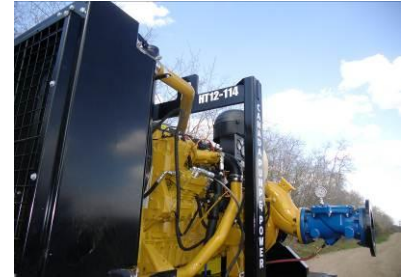
March – Pumps at Fire Water Pump House
